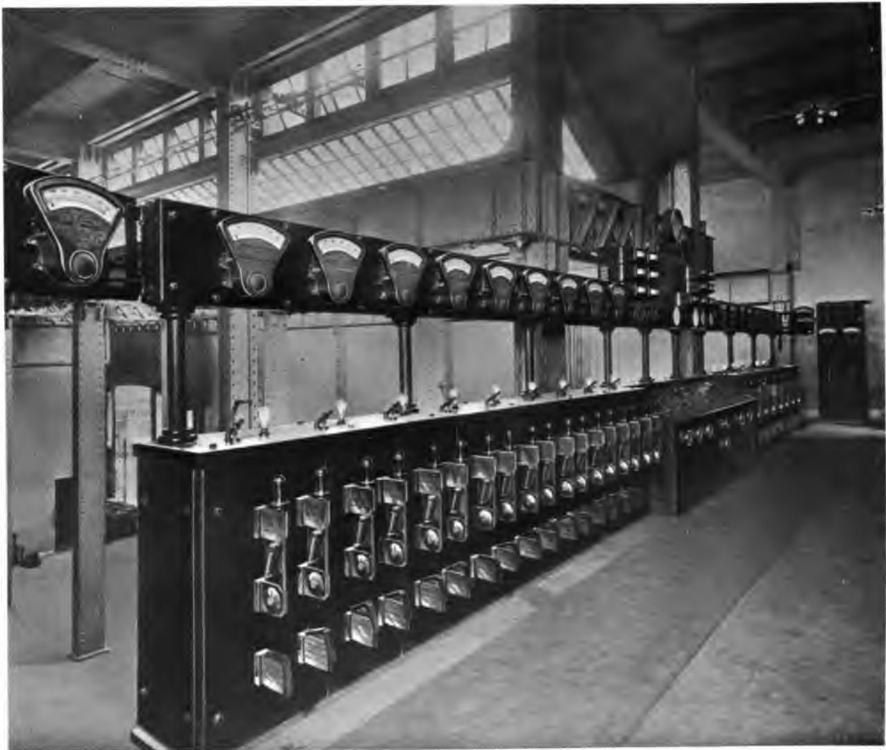
OPERATING BOARD—SUB-STATION NO. 11
